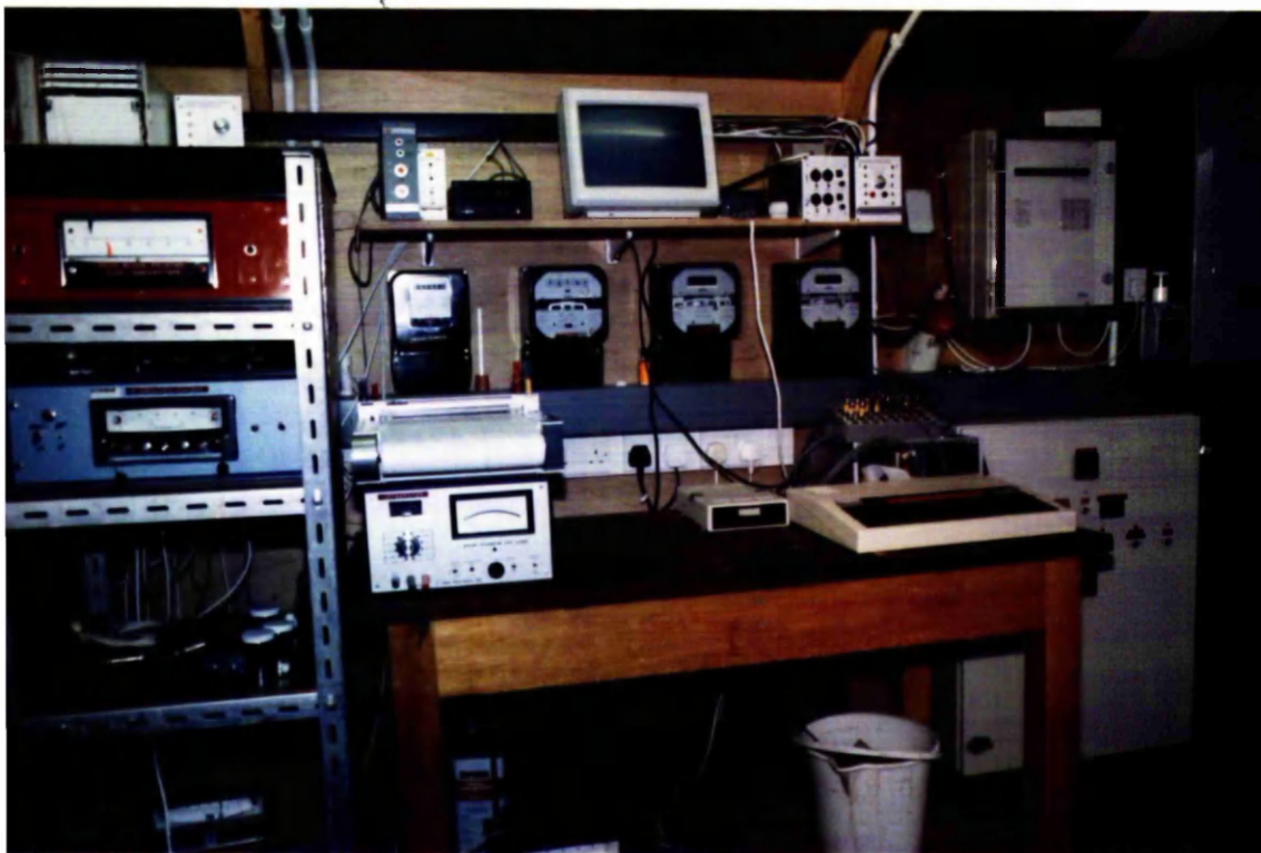
Fig.12 The plant control room.
