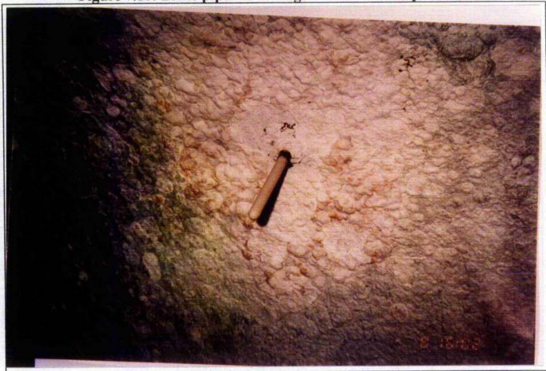
Figure 7.17: Seawater cooling water inlet (see figure 7.12)
