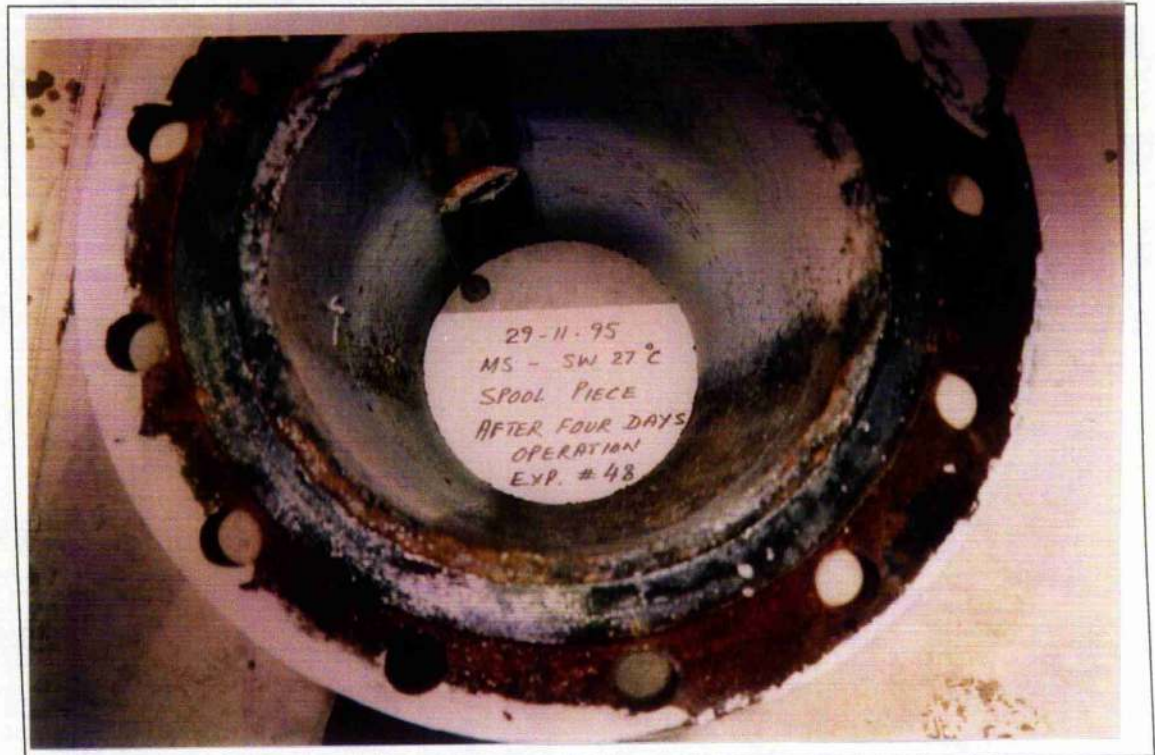
Figures 8.74 and 8.75: Specimens and spool piece condition.
