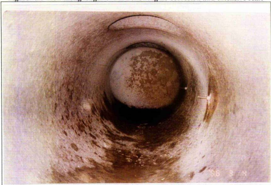
Figure 7.10: View along length of BIM showing no corrosion and extensive scale
