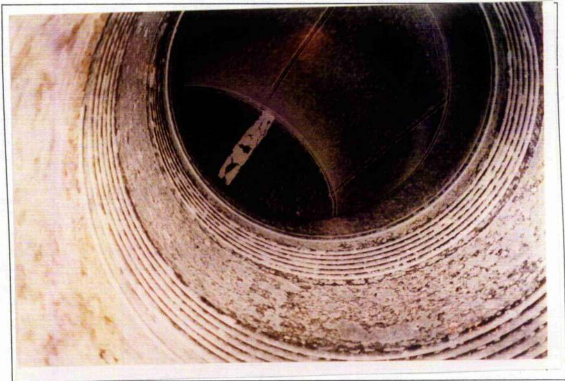
Figure 7.4: Photo of seawater internal pipe surface at the expansion bellow
