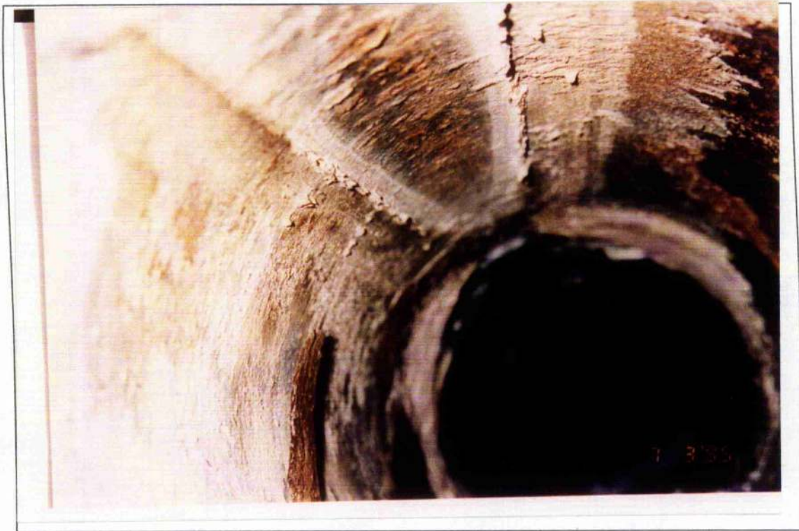
Figure 8.12: Scale built up on the surface of the test loop pipeline
