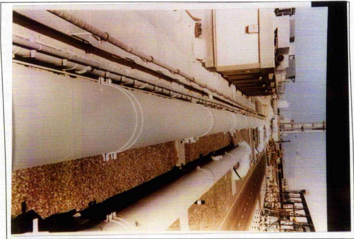
Figure 7.2: Photo of two seawater headers running parallel to evaporators
