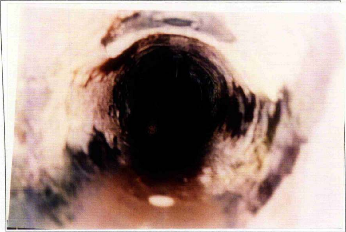
Figure 8.32: Pipeline condition at the end of test 29.
