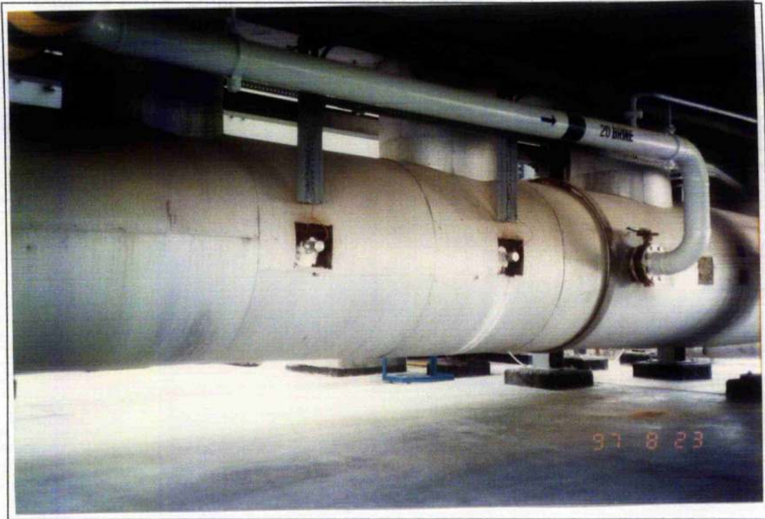
Figure 7.6: Photo of brine inlet manifold along with interconnection pipelines to flash chamber and also shows the 4 anodes installed in B.I.M
