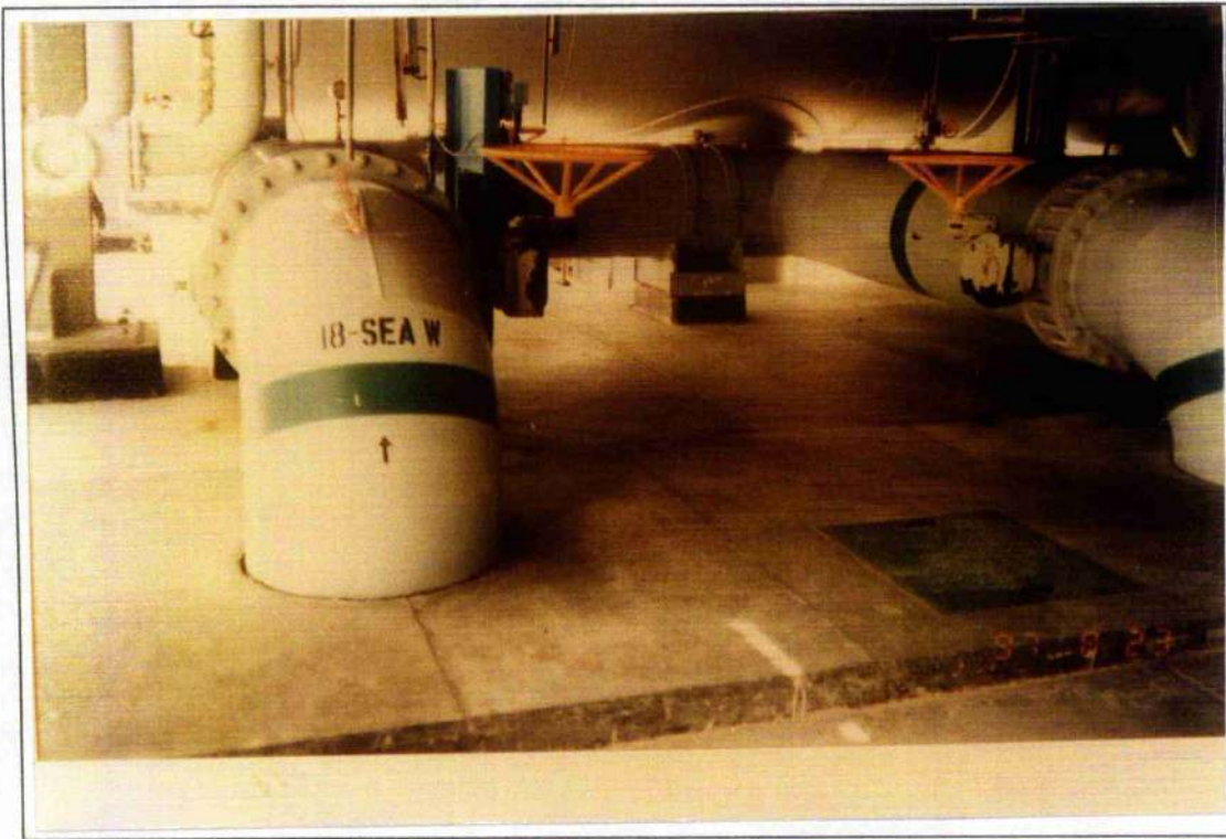
Figure 7.14: Photo of evaporator feed line
