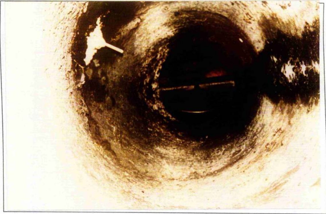
Figure 7.18: seawater cooling water outlet (see figure 7.13)
