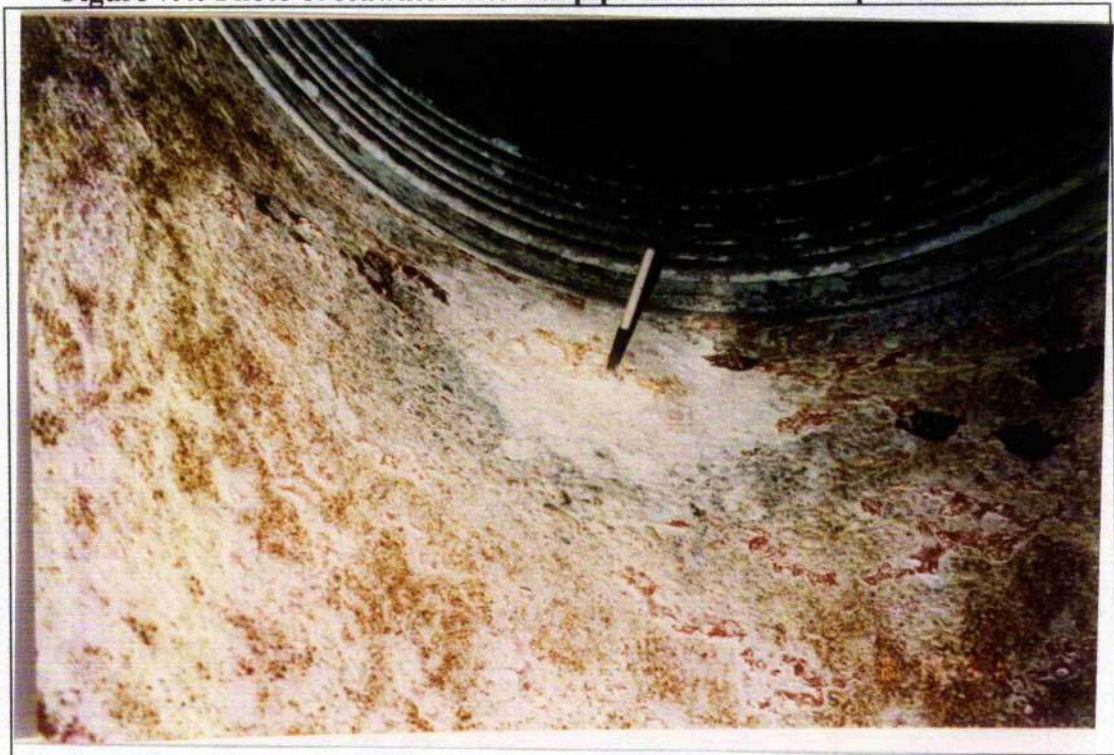
Figure 7.5: Photo of seawater internal pipe surface next to expansion bellow
