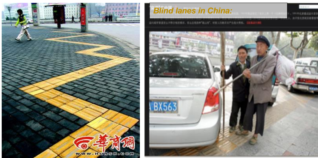
Picture 2-2 Poorly-designed and blocked blind lanes
