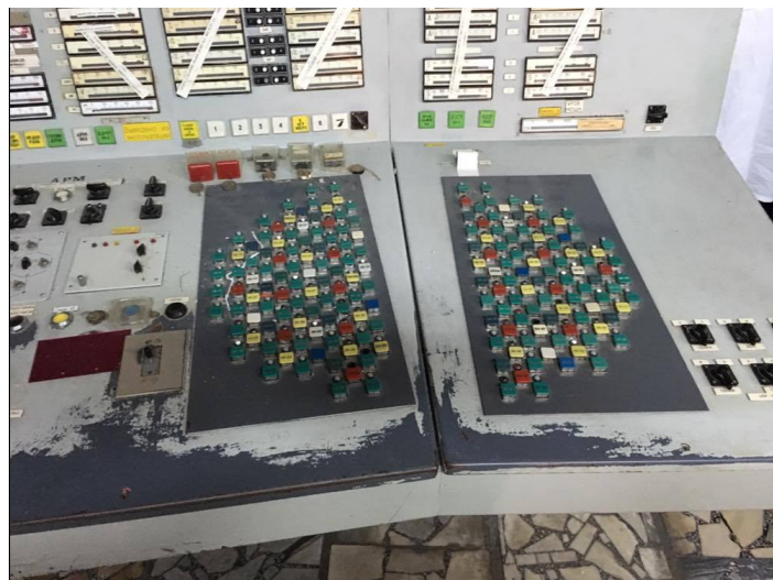
Figure 7.3 Retrofitted control panels within the control room of Unit 1 of the Chernobyl facility. (source: researcher's own photograph 2015)
