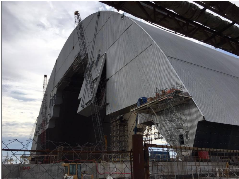
Figure 7.4 The construction site of the new containment structure. (source: researcher's own photograph 2015)
