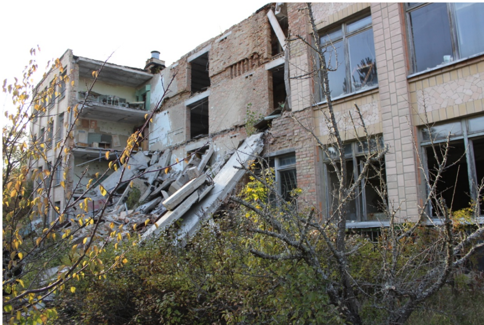
Figure 1.5: A collapsed School in North West Pripyat (source: researcher's own photograph 2015)
