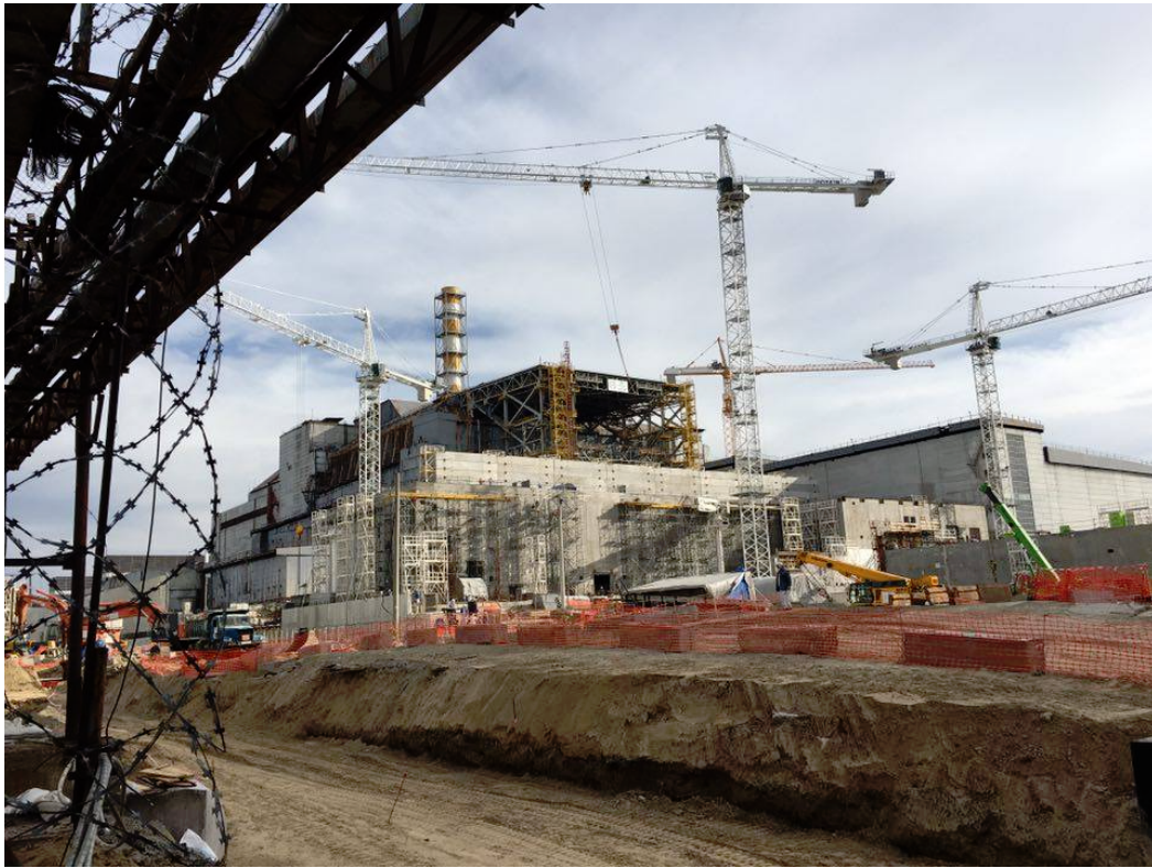
Figure 1.17: As close as one can get to the external wall of RBMK no4 (source: researcher's own photograph 2015).
