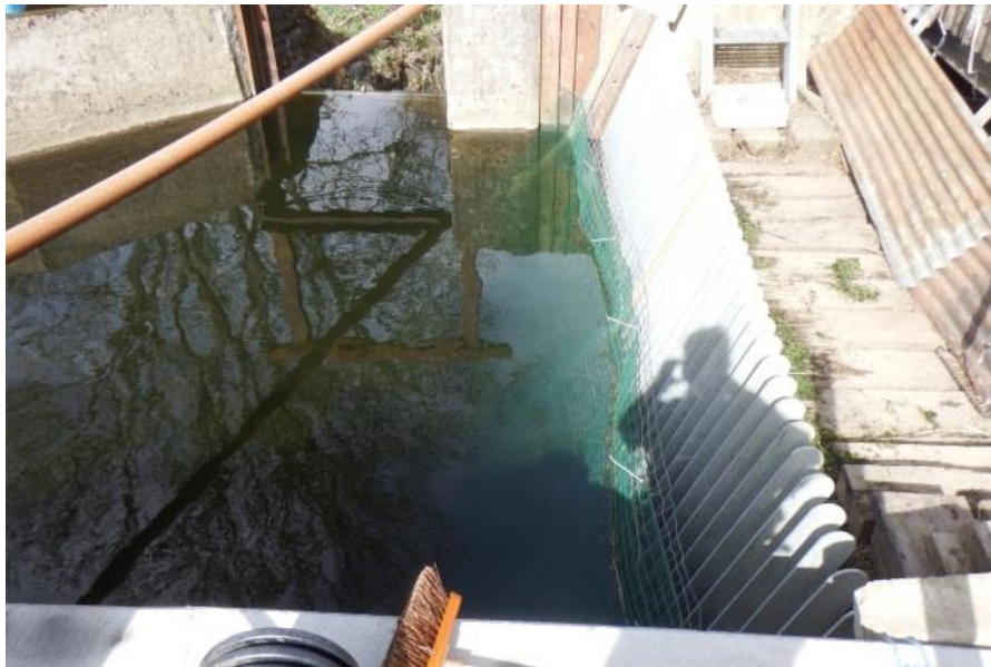
Figure 3.2. View of the upstream fence laid over the trash rack at the turbine intake in order to prevent fish escapement upstream and the entrance of wild fish during the trials.
