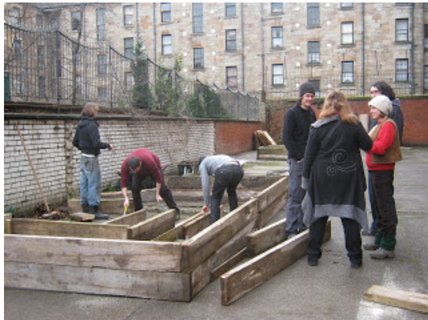
Plate 10: The doers in action. GSC participants aiding a community centre group in the construction of a community garden on the community centre grounds.
