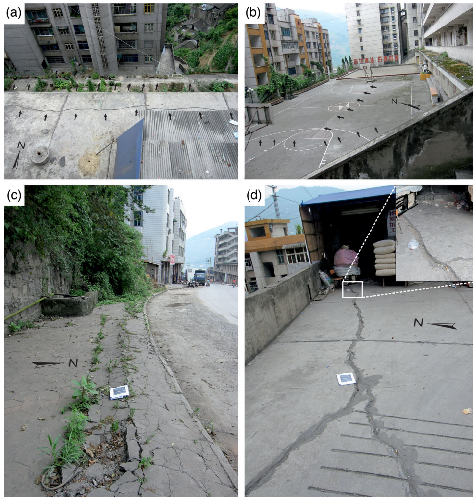
Figure 3. Cracks in Badong caused by the Huangtupo landslide. Note that north arrows, which approximately indicate the downhill direction, have been shown in the pictures.
