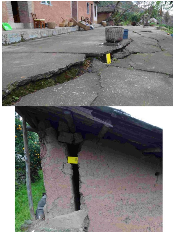
Figure A-4: Building damage indicative of land movements and confirmed in communication with residents. Photos were taken on 4 th April 2012 and located at 30° 59' 31N 110° 36' 41 E. The longest edge of the yellow notebook is ~0.16 m.
