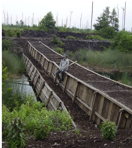
Figure 6.5 Large dam constructed across a drainage canal in degraded peatland in Block C, Mega Rice Project area. A timber frame was sealed with plastic sheeting and then filled with peat, adapted from Jaenicke et al. (Jaenicke et al., 2011).
