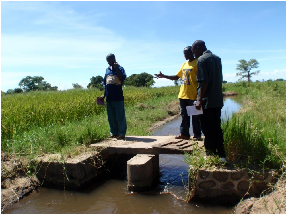
Picture 4.14: The Sakalilo irrigation scheme. This is being constructed to supply around 200 farmers with water throughout the year.
