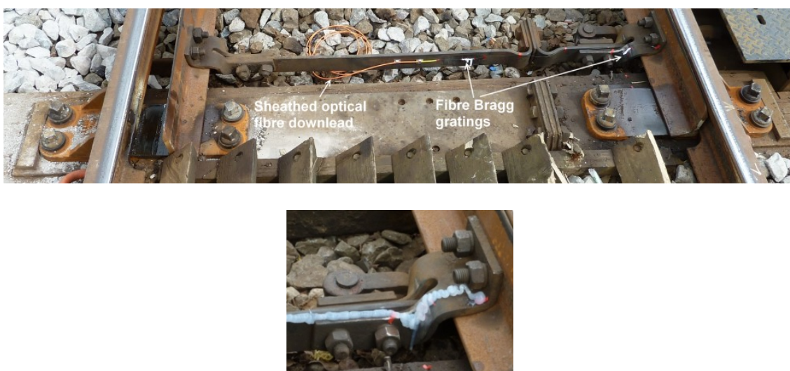
Figure 15. Images showing the placement of sensors on the stretcher bar and subsequent sealant protection.
