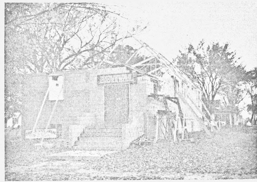
THE MINISTERIAL FELLOWSHIP project this year is the completion of this Nazarene Church Building in Momen, Illinois.
