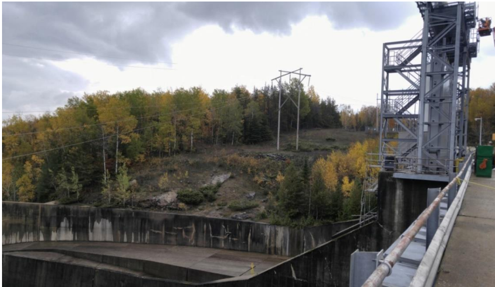
Fig.88: Side view of the sluiceway and sluice gates of Mountain Chute dam
