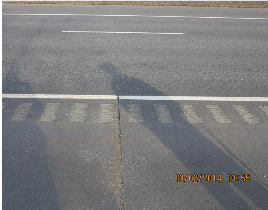
Figure 10. Precut active crack at ~ Station 1036+31
