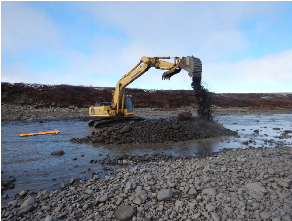
Figure 139. Digging the wet pit at the Sagavanirktok River near MP318 (DSS4) on September 15, 2015 (from Toniolo et al., 2016b).
