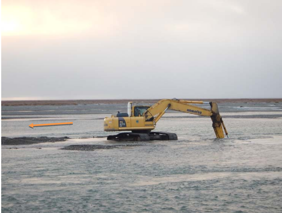
Figure 127. Digging the wet pit at the Sagavanirktok River near MP405 (DSS1) on September 9, 2015 (from Toniolo et al., 2016b).
