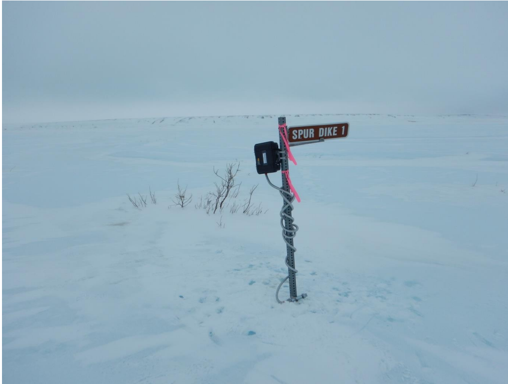
Figure 3. Water level sensor installed at spur dikes near Franklin Bluffs to monitor water levels from overflow and spring breakup.
