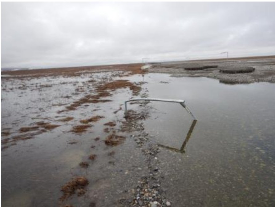
Figure B.16. Photo taken May 26, 2015, near Dalton Highway MP395, view south. Water has stilled and cleared, revealing the depth of damage to the road. Bent delineator noted in Figure B.15 was the location of a water-measuring instrument that broke free during ice collision and was subsequently buried in deposited gravel west of the road. Unfortunately, the instrument was not recoverable.
