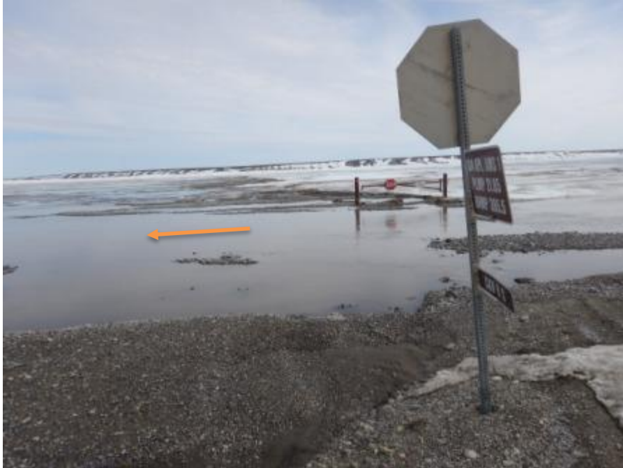
Figure B.13. Photo taken May 21, 2015 at Dalton Highway MP395.5, view east. Photo shows access road rendered impassable until repair. Water levels are falling, and although most of the ice has melted in the foreground, a considerable amount remains in the area beyond the gate.
