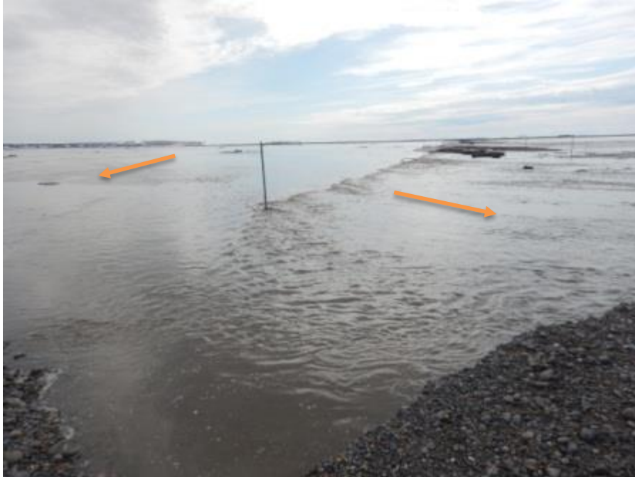
Figure B.15. Photo taken May 21, 2015, near Dalton Highway MP395, view south. While some ice remains under the water on the left, the road has been eroded down to the underlying tundra. Note the bent delineator, above and right of photo center; this is the left-most delineator in Figure B.14. This delineator was hit by large mobile ice transported in the current by sliding on top of the aufeis.
