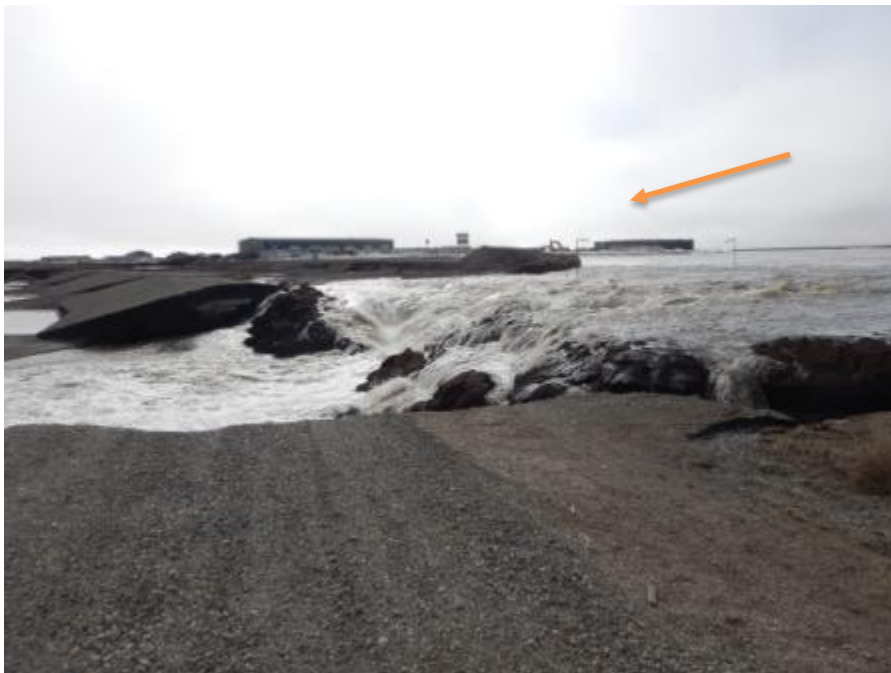
Figure B.2. Photo taken May 20, 2015, near Dalton Highway MP414, view south. Dark material is permafrost.
