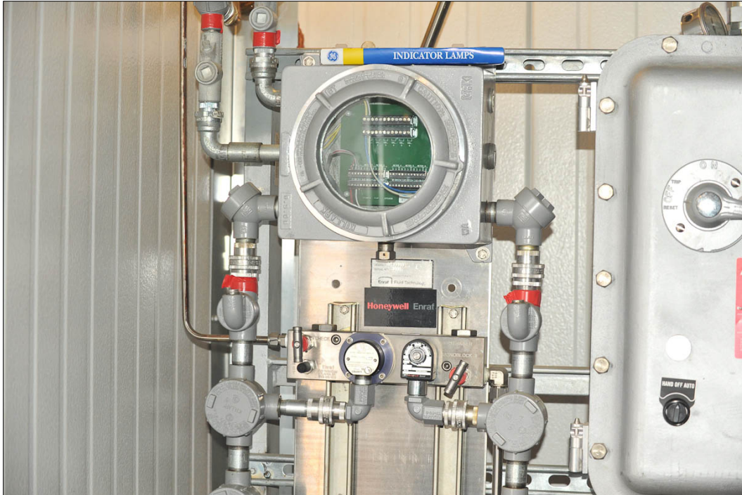
Figure 10. Blending meter for lubricity additive, PetroStar Refinery, North Pole, Alaska. Lubricity additive is precisely and accurately metered and pumped with electronic control for injection into the diesel fuel that is pumped into delivery trucks outside. Photo by Frank Williams.
