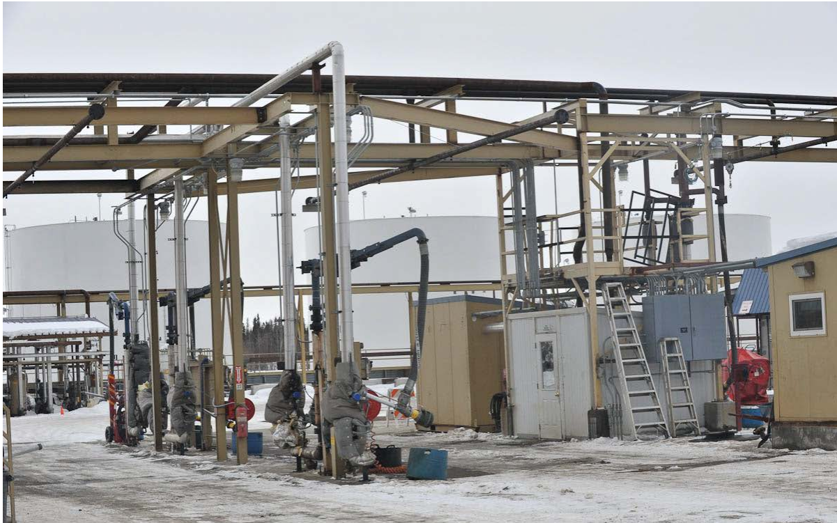
Figure 9. Diesel fuel delivery station at PetroStar Refinery, North Pole, Alaska. The gray building just to the right of center houses the metering and injection of additives. Truckers enter orders for fuel and fuel blends in the brown building at the front right of the gray building. They use an advanced control and metering system for dispensing the requested fuel into delivery trucks positioned in the station. Fuel storage tanks can be seen in the background. Photo by Frank Williams.
