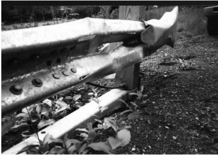
Fig. 1 Damage to the Slotted Area in W-beam of SRT-350s
