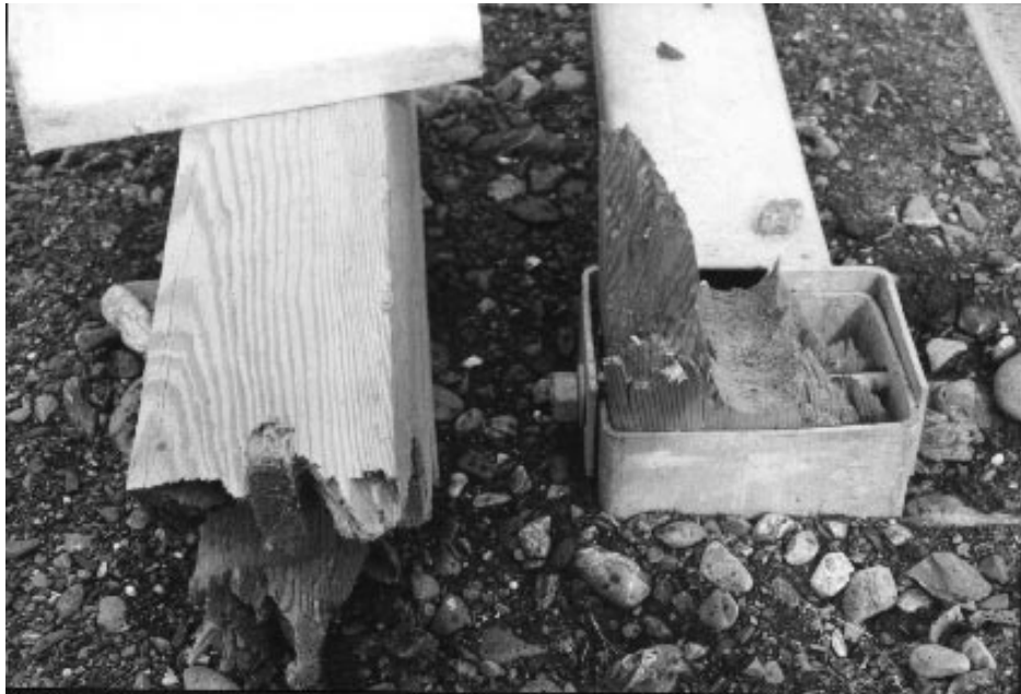
Fig. 3 Wooden Post Broke away from Its Steel-Tube Base
