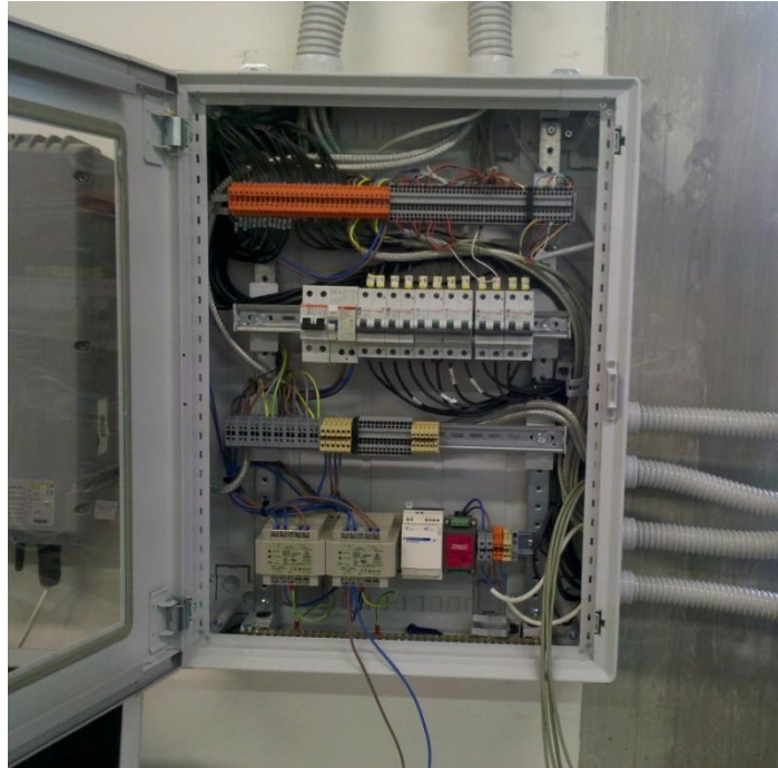
Figure C. 4 Electric switchboard in the power system lab
