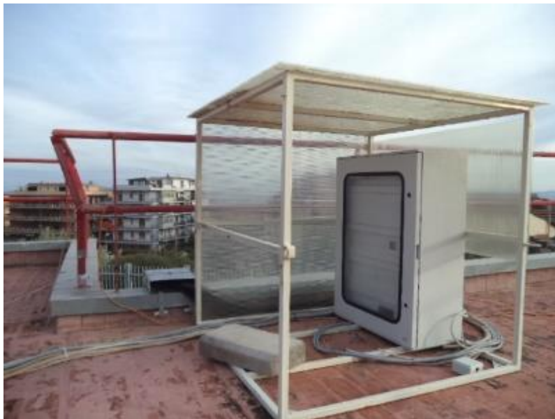
Figure C. 3 Switchboard installed on the roof of the power system lab
