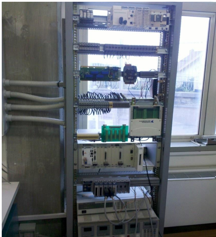
Figure C. 5 Rack that lodges appliances, terminals and wiring
