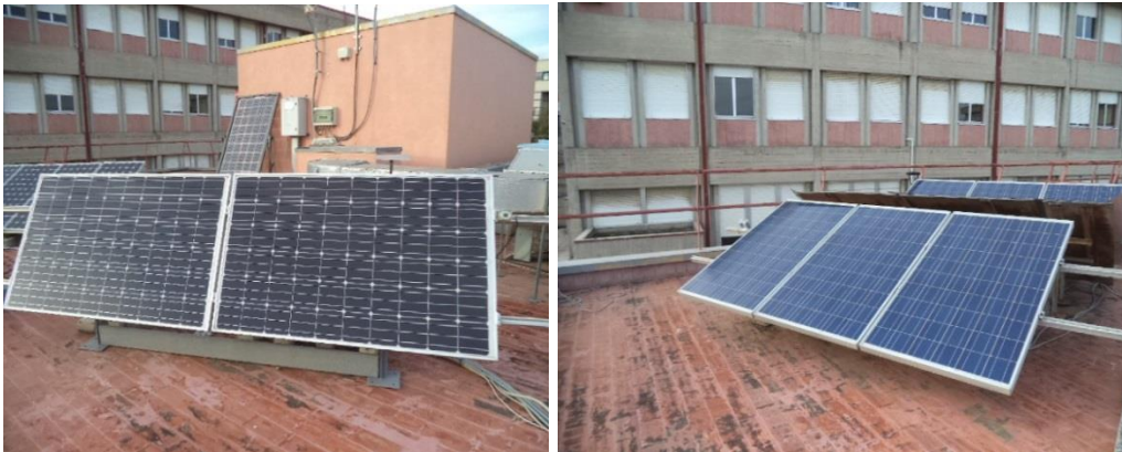
Figure C. 1 PV module installed on the roof of IDRILab building: single PV modules (left), PV string (right).
