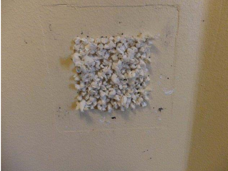
Figure 15: Inmate cell vent filled with toilet tissue for thermal and sound control
