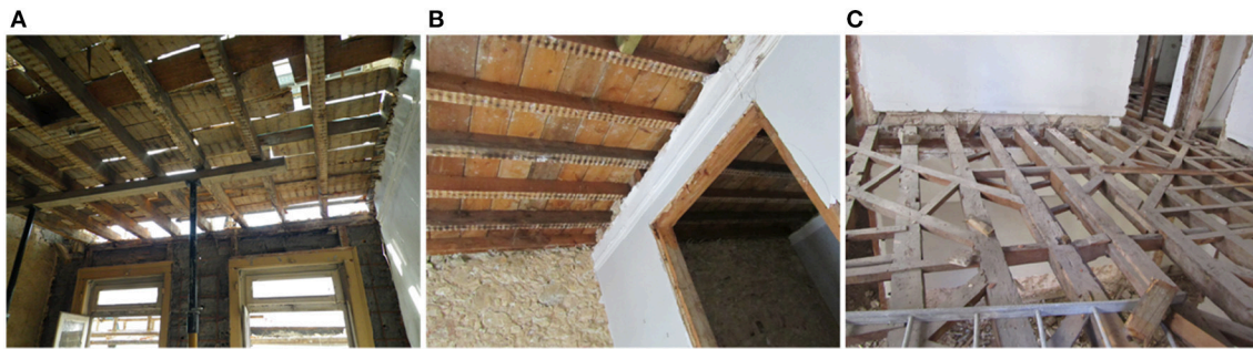
FIGURE 6 | Masonry walls with different type of materials: (A) Rubble stone, (B) Brick, and (C) Concrete block.
