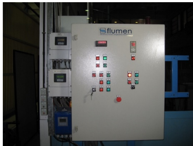
Figure 3:7 Electronic control of hydraulics pumps
