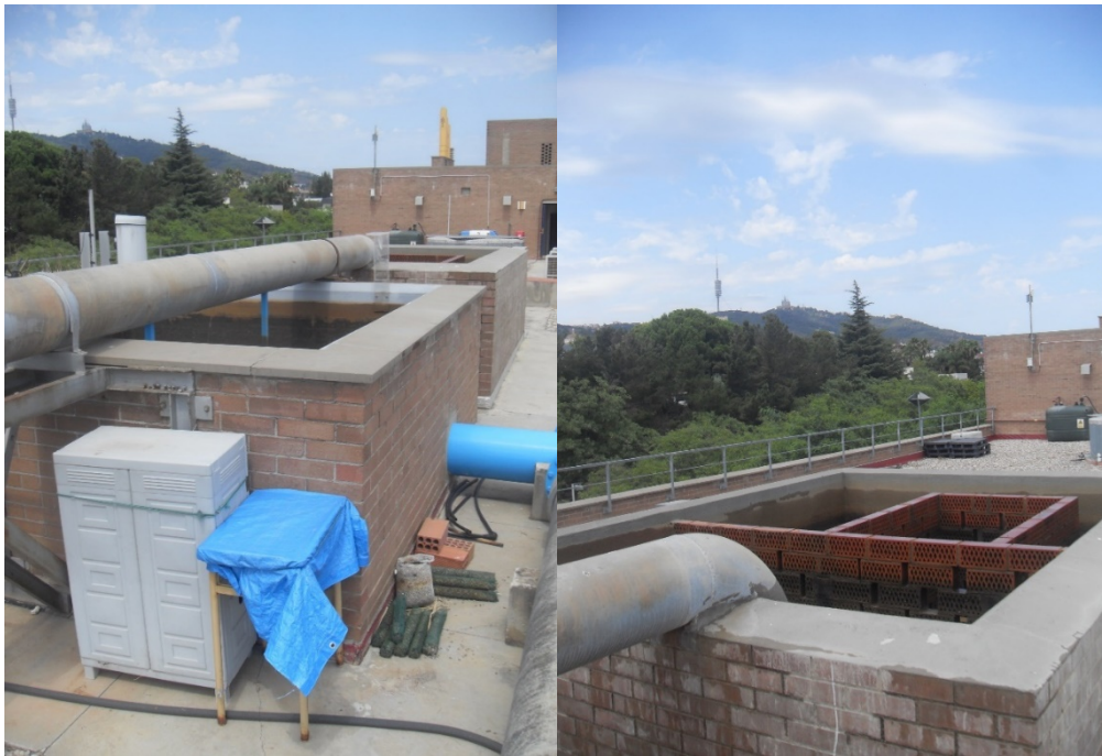
Figure 3:6 Reservoir tank located at the roof of the building
