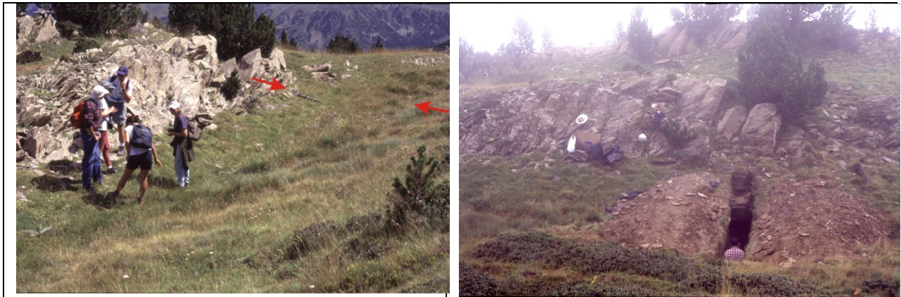
487 Fig. 11. Site of trench 3. (a) Left, site before trenching, view to NE. Trench was dug between two red 488 arrows. (b) Right, view of trench 3 looking N. 489
