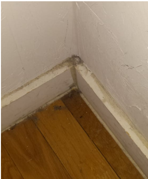
Figure 32: Dirt in corner of a room.
