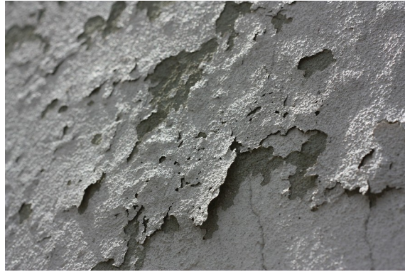
Figure 25: Peeling effect on a wall. See how the layer beneath is visible through the holes in the upper one.
