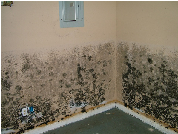
Figure 26: Mold stuck on a wall.
