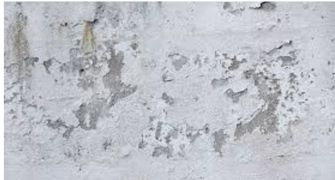
Figure 111: Real picture of peeled wall.
