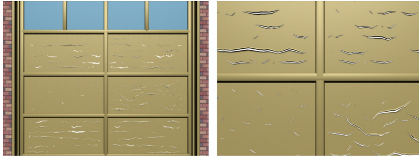
Figure 5: [PPD02] peeling approach.
