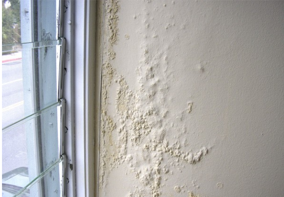
Figure 107: Real picture of wall humidities
