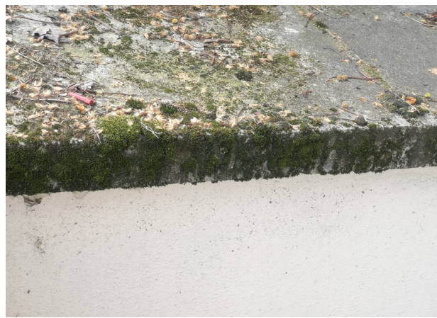
Figure 27: Moss in a building made of rock.
