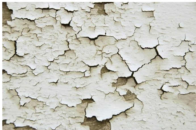
Figure 113: Real picture of peeled wall.
