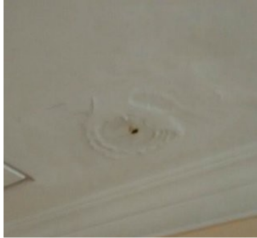
Figure 31: Humidity in ceiling.
