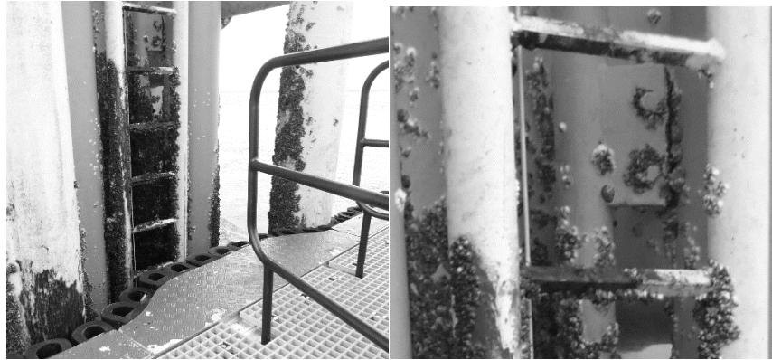
Figure 2a & 2b: Examples of the external ladder on a turbine. NB.
