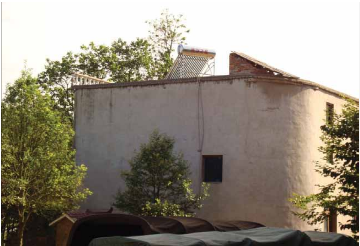
Figure 14. Solar water heaters installed in the watershed farmers houses.
