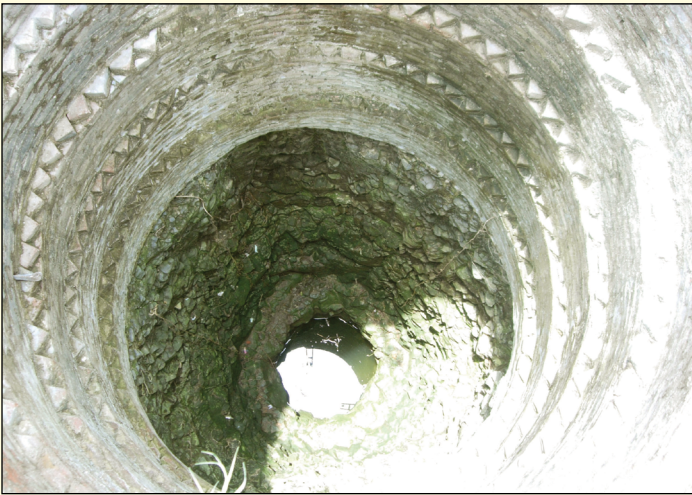
Wells get deeper and drier as exploitation of ground water increases, India.
