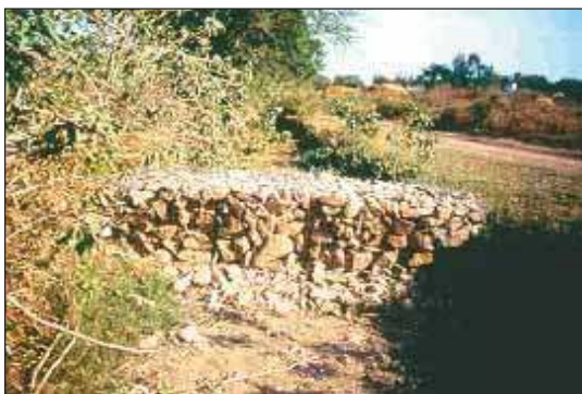
Figure 11. Rock reinforced with wire mesh and steel posts for controlling gully in Lalatora watershed, Madhya Pradesh, India.
