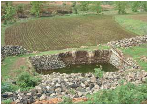
Figure 25. A defunct well recharged after construction of check-dam and more area brought under cultivation in Dewas, Madhya Pradesh, India.
