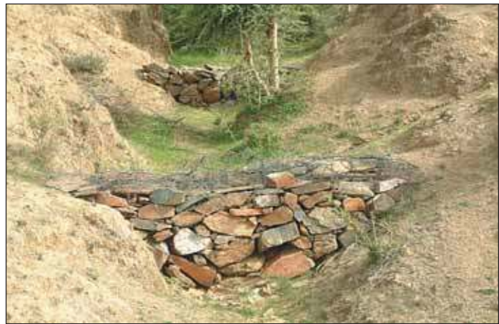
Figure 17. Series of stone wall dams for controlling gully in Bundi, Rajasthan, India.
