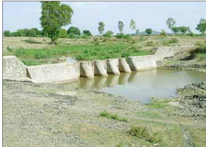
Figure 20. Masonry check-dam with additional support for stability in Madhusudhangadh watershed, Madhya Pradesh, India.
