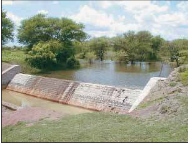
Figure 18. Masonry check-dam for controlling gully and water harvesting in Adarsha watershed, Kothapally, Andhra Pradesh, India.
