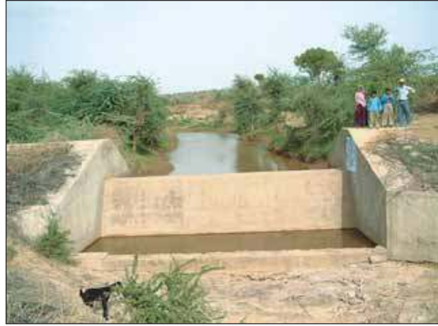
Figure 19. Masonry check-dam for controlling gully and recharging groundwater in Bundi, Rajasthan, India.
