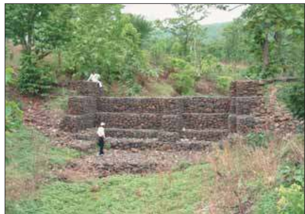
Figure 27. Gabion structure across a big nala in Dewas watershed, Madhya Pradesh, India.
