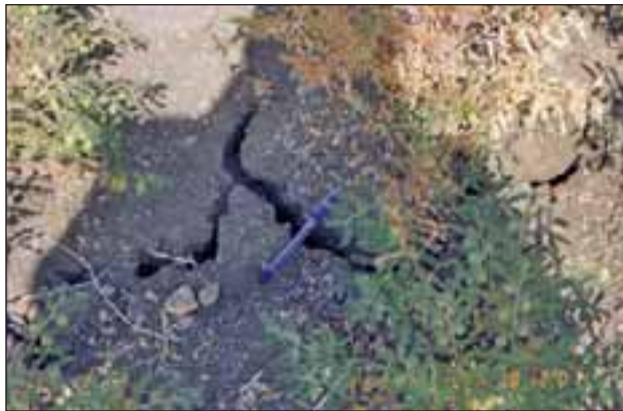
Wide and polygonal surface cracks in the benchmark spot
