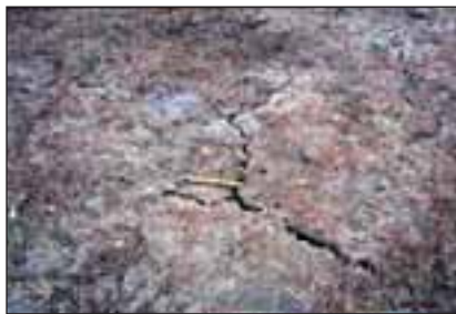
Wide and polygonal cracks in benchmark site at Jajapur
