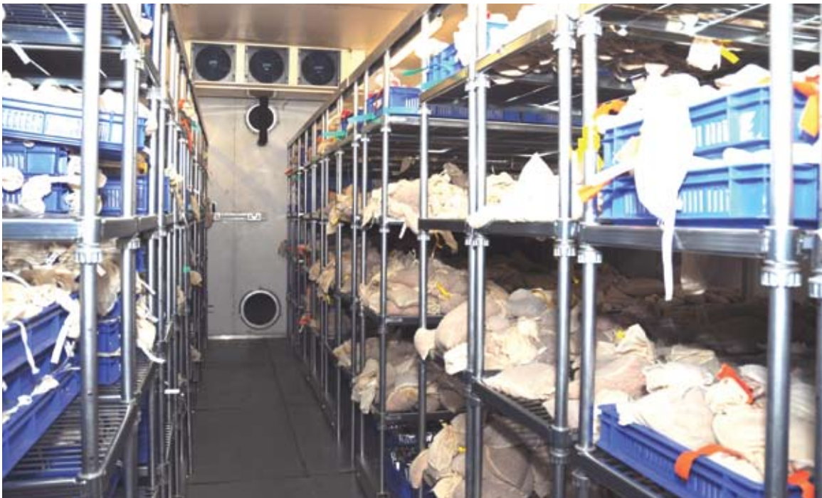
Figure 4C.1.2. Walk-in seed drying room at ICRISAT genebank.
