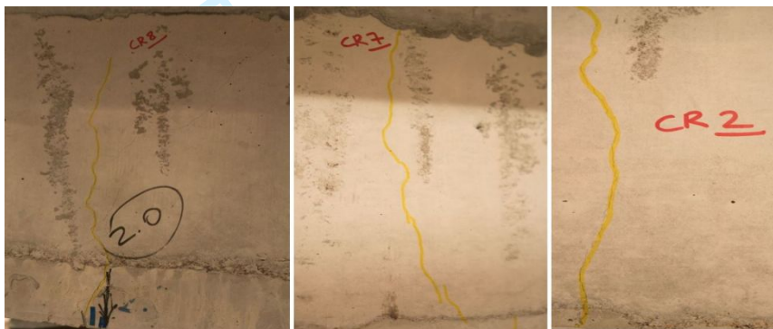
6 7 Figure 2. Detected cracks on body of the BGB in damaged state.
