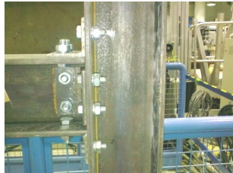
(d) Beam-column connection on the right hand side of the first storey
