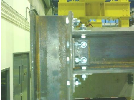
(a) Beam-column connection on the left hand side of the second storey
