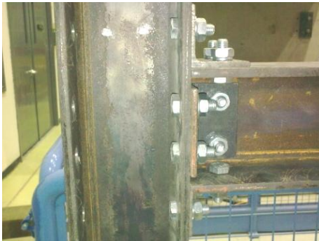
(c) Beam-column connection on the left hand side of the first storey
