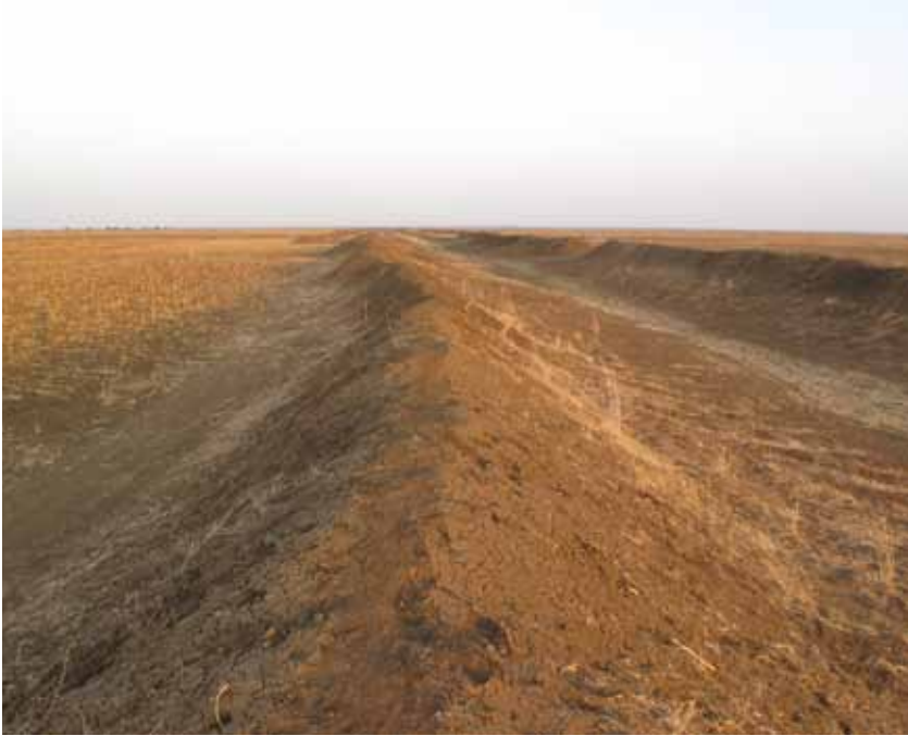
706.jpg: The newly excavated canal. It is yet unconnected. The eastern end is at the railway line near the main road, before it reaches the Blue Nile.
