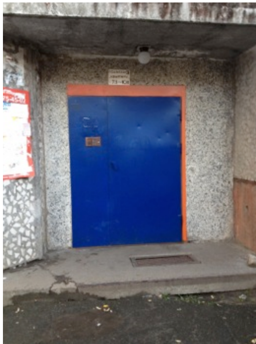
Figure 22: A typical entrance doorway in the Drevlyanka region of Petrozavodsk. Notice the uneven ground and disrepair of the stoop, and the idiosyncratic paint on the metal doorway.
