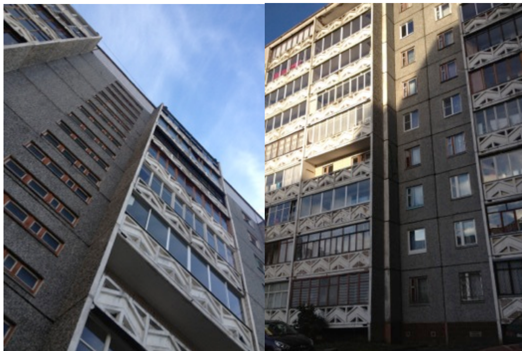
Figure 20: Photos of housing in the Drevlyanka region of Petrozavodsk. Buildings in this region are from the series built in the 1980s; Notice the graphic element of design in the balcony paneling that is specific to this region of the city. My photo.
