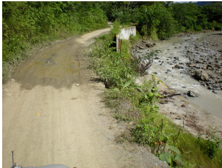
Figure 19. Nearing San José de Apartadó on the road from Apartadó. During heavy rains, there are frequent landslides, one of which pushed the retaining wall seen here (financed by the presidential development agency Acción Social ) into the Río Apartadó . The Apartadó River flows down from the Serranía de Abibe and provides water to Apartadó and the banana plantations in Urabá's lowlands. Source: Author photo.
