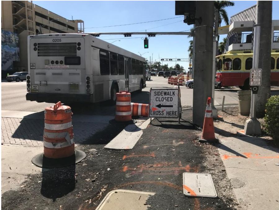
Figure 5.4. The public pedestrian experience along Broward Avenue in Fort Lauderdale, immediately adjacent to the public bus terminal. Chaos and cones. “Sidewalk Closed”, beg buttons, and an 8-lane stroad to cross. ADA-non complaint. Ignorant of the pedestrian experience.
