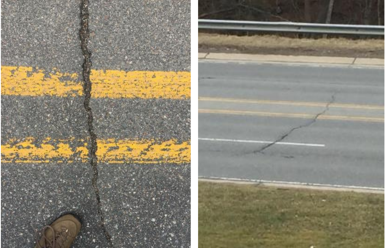
Figure 16: Crack propagated through Highway 321 from Aug 2013 earthquake.
