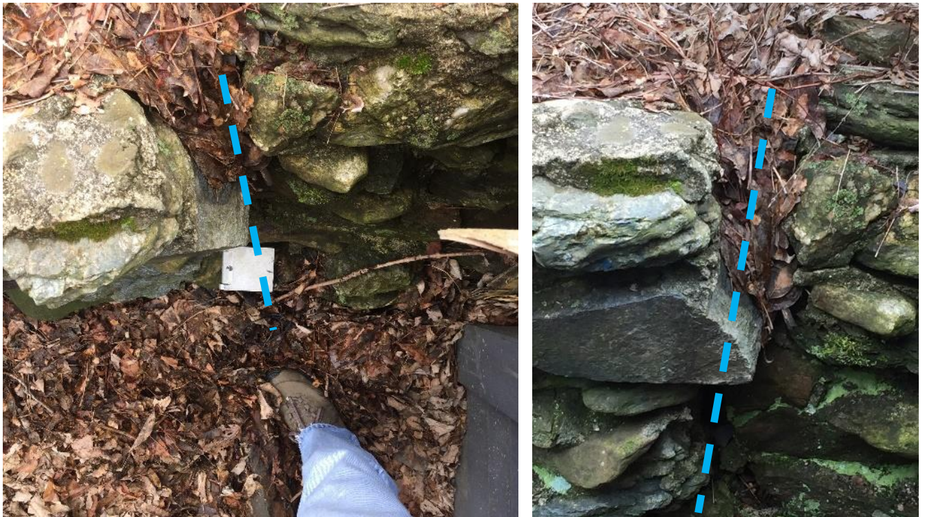
Figure 14: Aerial and frontal views of the cracked retaining wall behind Doc’s Rocks storefront. Damage from Aug 2013, photos from Feb 2019.
