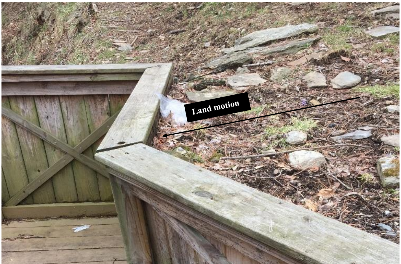
Figure 15: Displacement of stairwell fence from damage of Aug 2013 earthquake.
