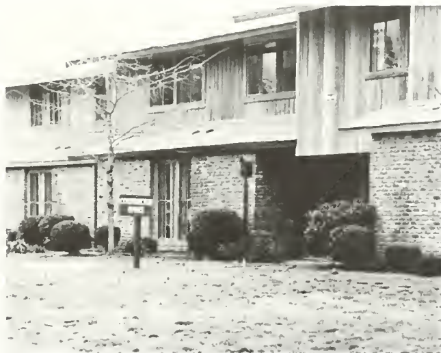
Repairs on condominiums are often only of an exterior, cosmetic nature. Photo by John Gaadt
