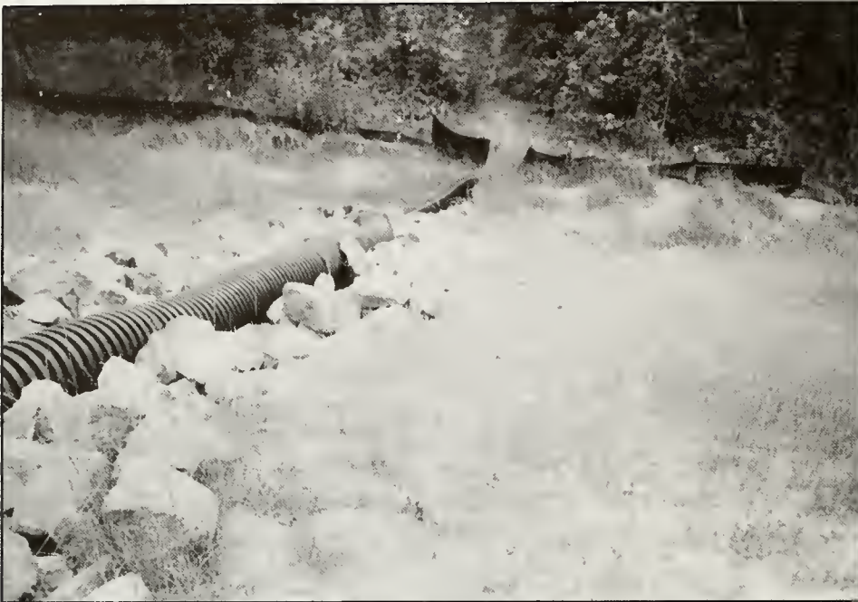
Good practice: A slope drain, anchored in rip-rap, channels run-off to where it won't erode the slope.
