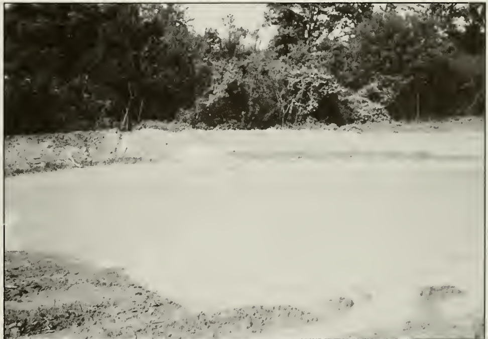
Good practice: A well-designed sediment pond includes a vertical riser and trash guard.
