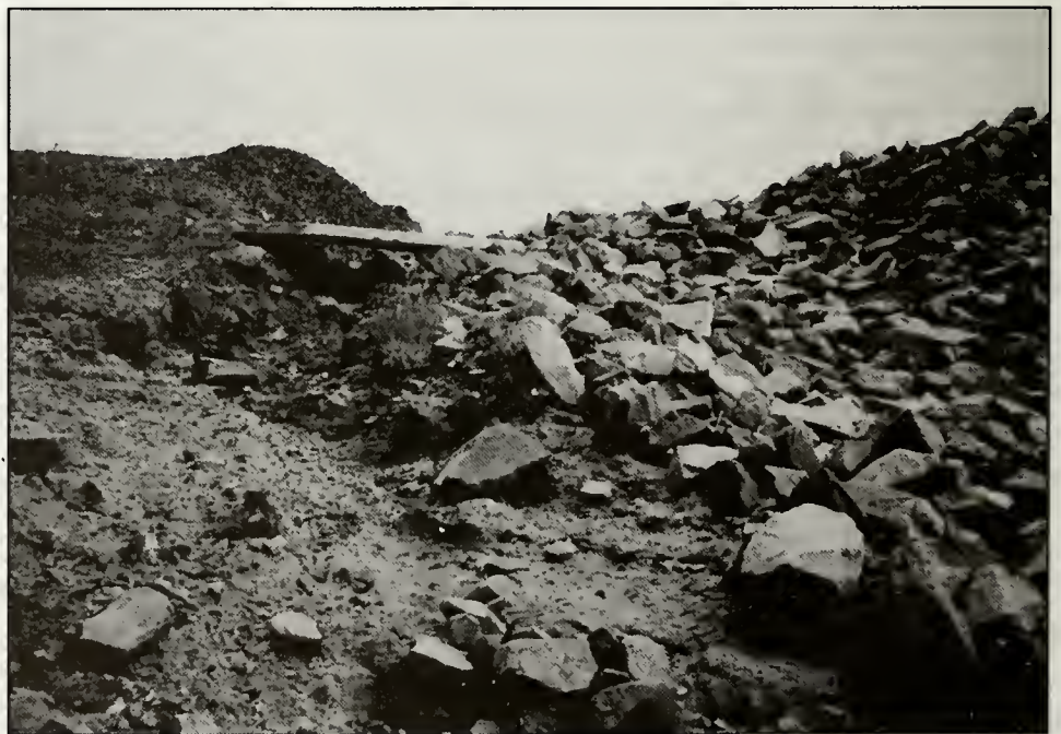
Bad practice: A rip-rap channel, designed to filter out sediment, is ineffective because a trap failed, allowing water to bypass it.
