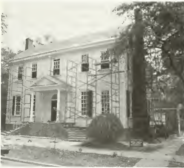
Restoration is currently taking place in the Tarboro, N.C. Historic District. Photo courtesy of E. Watson Brown, Town of Tarboro
