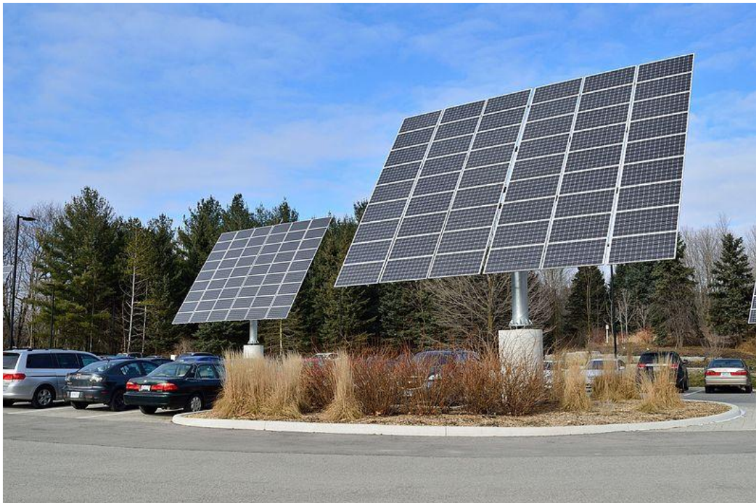
Figure 4 Solar modules mounted on solar trackers [25]
