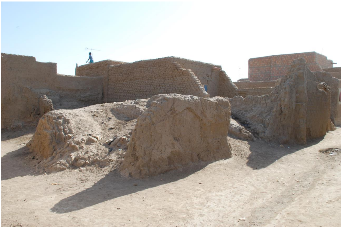
Figure 1-4: An example of damage sustained by an unstabilised earth building, which can suffer from low durability. Image courtesy of Prof. Pete Walker.
