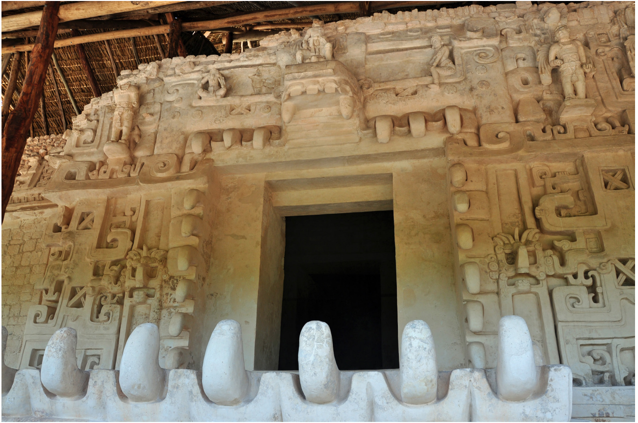
Figure 4.6. Entrance to burial chamber of Ukit Kan Le'k Tok' behind ornate white stucco façade on the Acropolis of Ek' Balam (photo by author).
