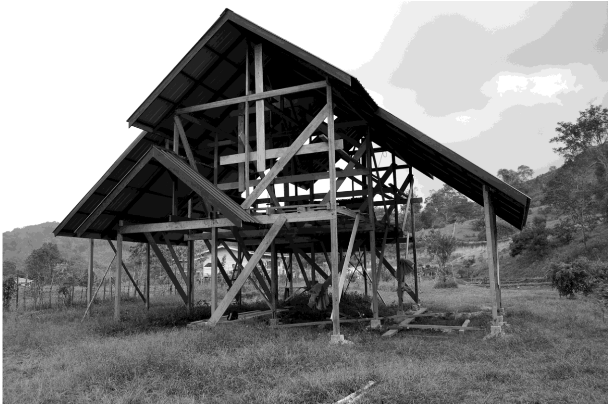
Figure 3: Modern housing: Individual house with 2 storeys; (green) painted aluminium roof with insulation under; metal and concrete foundations.
