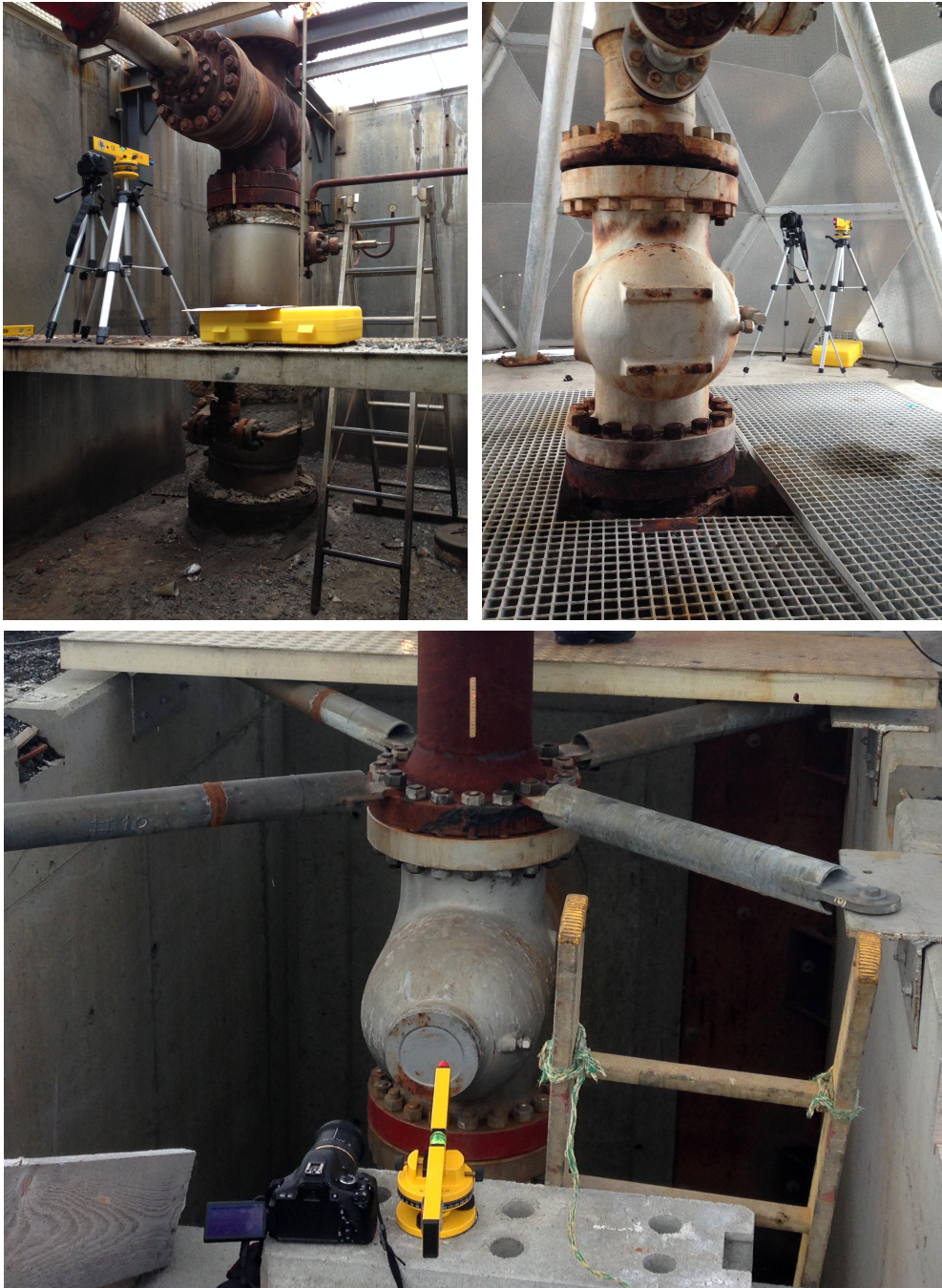
Figure 5.29: The setup and wellhead of wells RN-22 (top left), HE-53 (top right) and RN-32 (bottom). The laser is projected on a ruler above or below the master valve. For the HE wells the setup was similar to that of HE-53.
