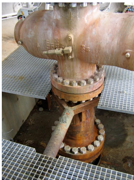
Figure 4: The expansion spool and master valve of the wellhead of well HE-46 (figure: Heimir Hjartarson).
