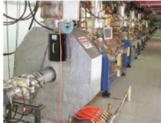
FIGURE 7. A 7.5 MHz Finemet rf cavity installed in the Fermilab Main Injector.
