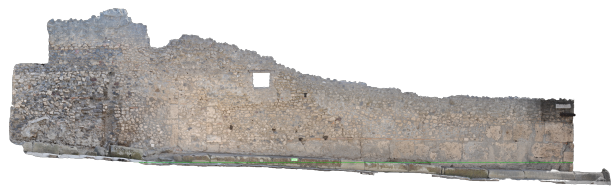
Figure 8. Ortho-photography of the west wall outside, extracted from the 3D model from terrestrial photogrammetry
