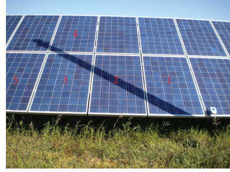
FIGURE 4: The numbers of the PV modules shaded by wire pole.
