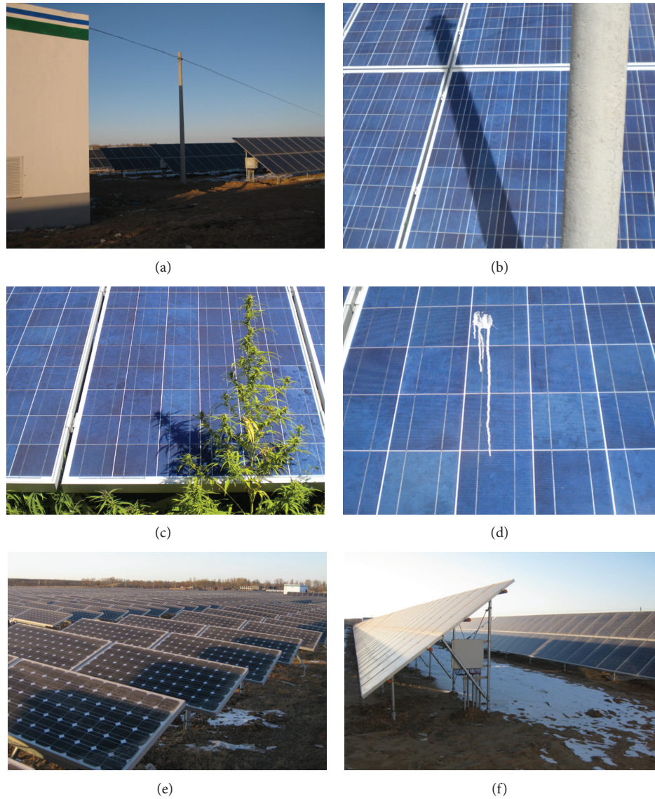
FIGURE 3: Different types of shading in a large scale grid-connected PV plant in northwest China. (a) Power distribution buildings shading; (b) wire poles shading; (c) plants shading; (d) bird droppings shading; (e) tracking PV system shading; (f) fixed PV system shading.
