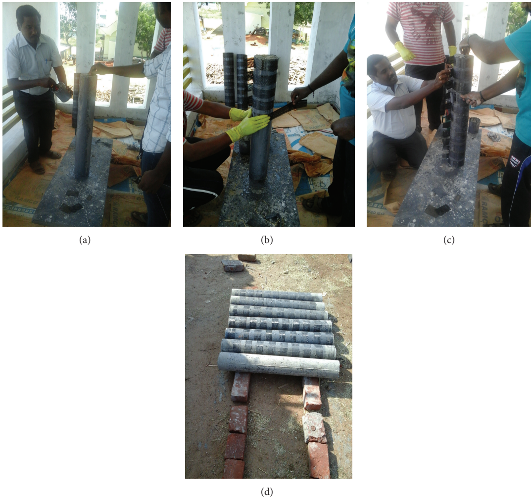
FIGURE 2: Wrapping procedure [55]: (a) applying resin coating; (b) wrapping CFRP strips; (c) removing excessive resin using steel roller; (d) all strengthened beams.
