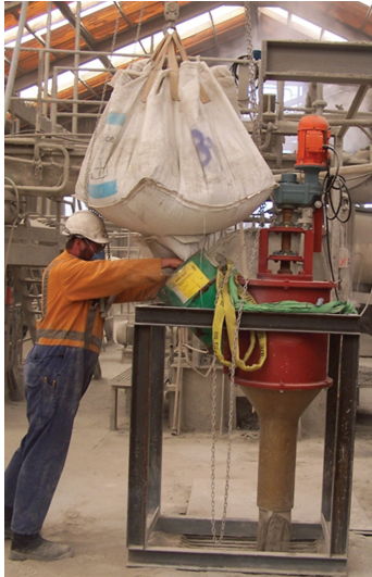
FIGURE 7: Advanced commissioning of vertical feed screw during plant operation. Image shows plant being fed with material via a temporary arrangement while being commissioned. (Photograph by K Lawry and used by permission of Ballance Agri-Nutrients.)
